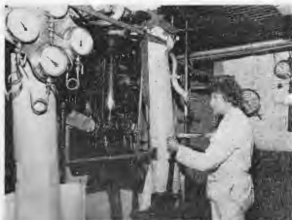
Main engine-room controls, under the hand of Taioma's Chief Engineer, Theo King.
